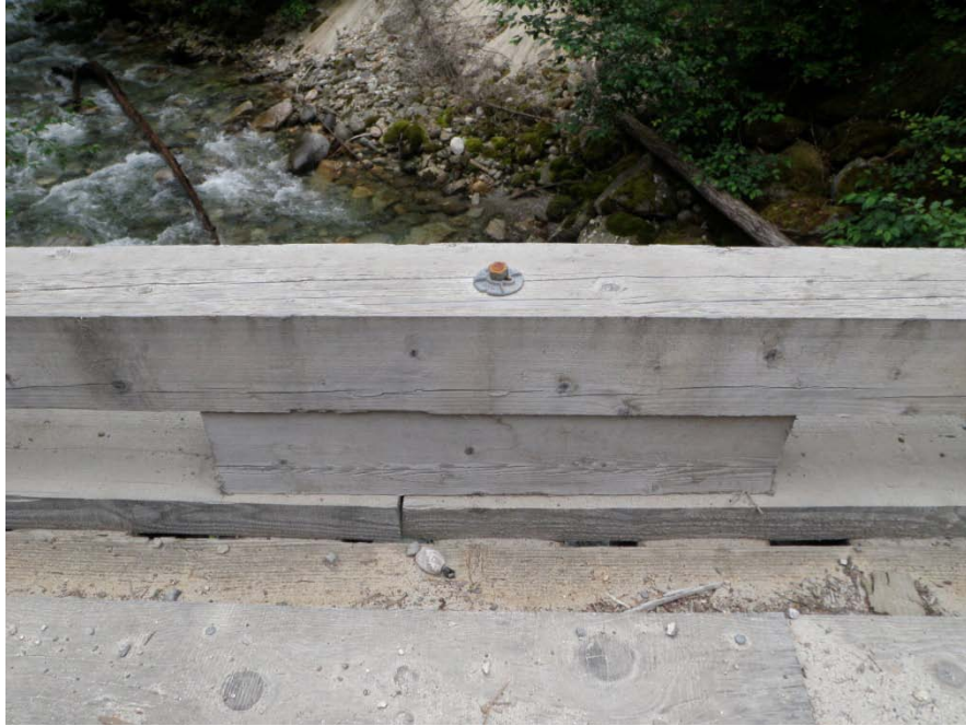
Riser and curb with only 1 bolt
